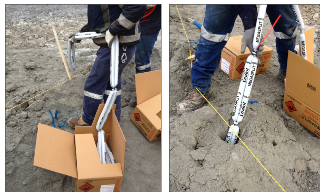
3. Withdraw base charge and feed down hole. Retain firm hold while feeding charge into hole.
